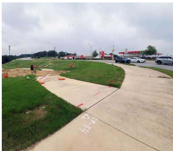
Trail segment under construction at Bulverde Rd and Classen Rd in San Antonio, TX
